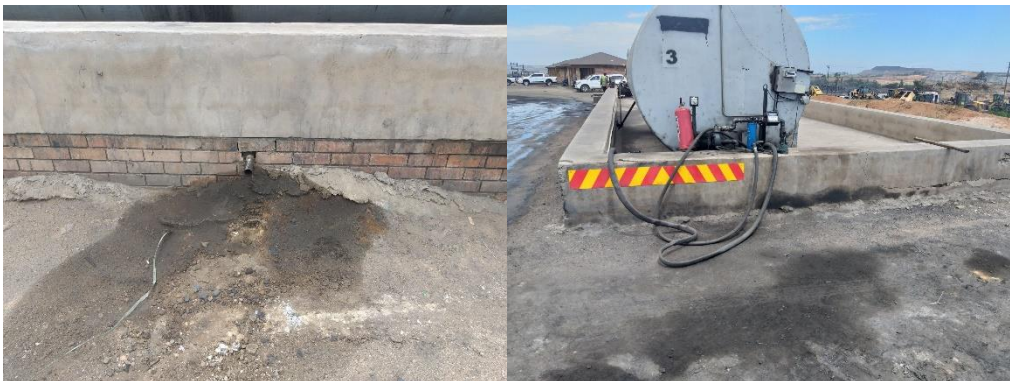
Figure 11: Lack of valve at the bund wall drain and seepage on the outside of the bund wall of the bulk diesel storage area adjacent to the workshop offices.
