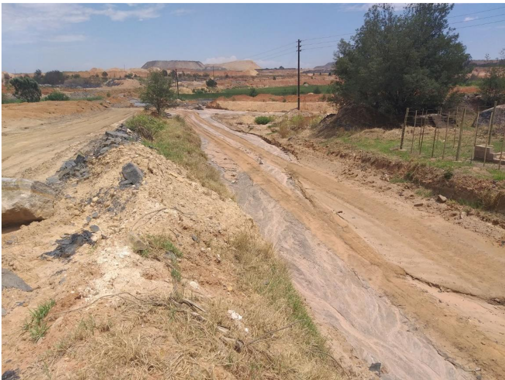
Figure 9: Erosion and silt wash on the access road leading to the watercourse.
