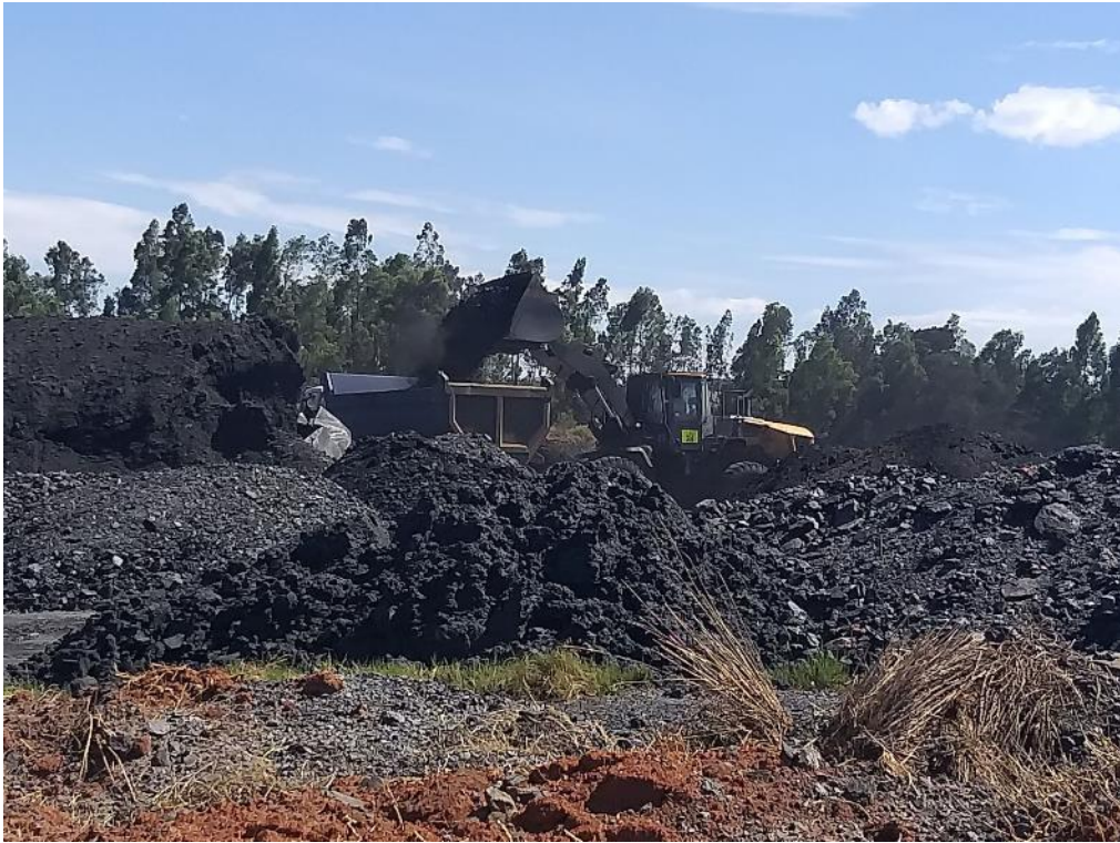
Figure 2: Removal and re-processing of the historically disposed discard within the pits in the northern section of the MR 314 MP Mining Right.
