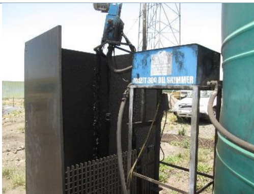
Figure 5: Oil-skimmer at oil-water separator system at the workshop.
