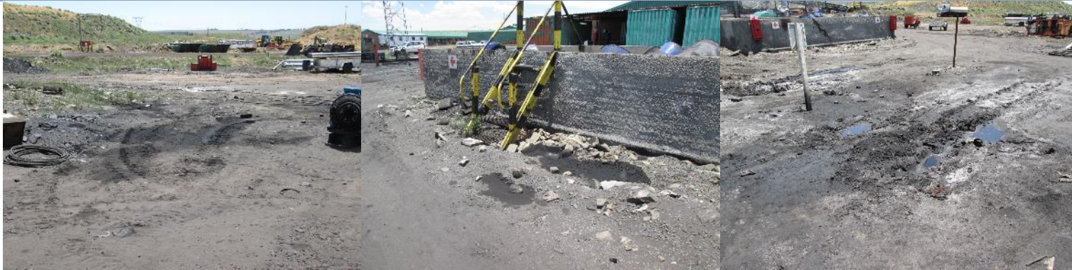
Figure 8:Hydrocarbon spillages noted during the audit.
