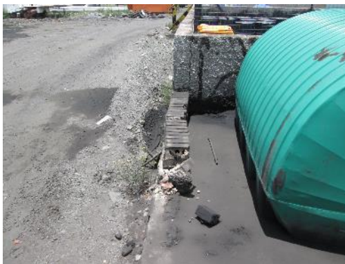
Figure 6: Broken bund wall at the laydown area.
