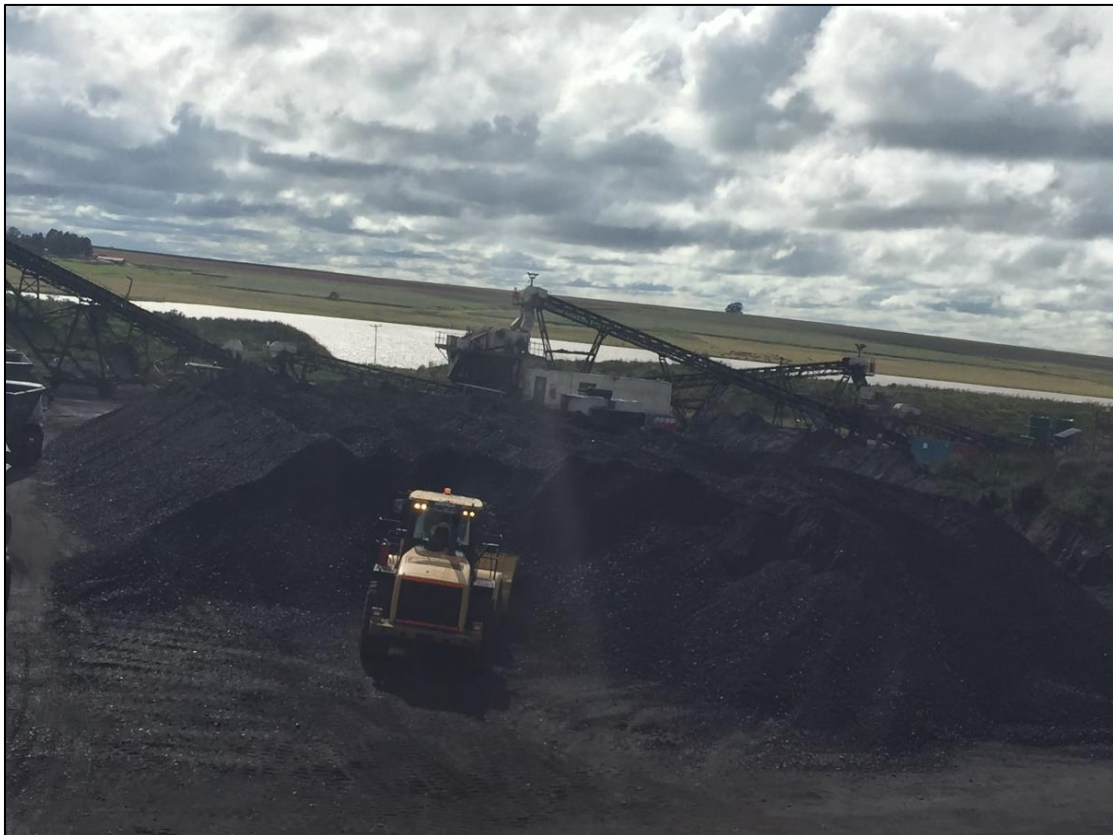
Figure 6-3: Manungu Crushing and Screening Plant
