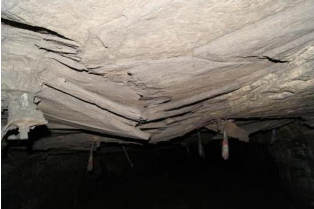
Figure 8: Underground roof buckling as a result of high horizontal stresses.
