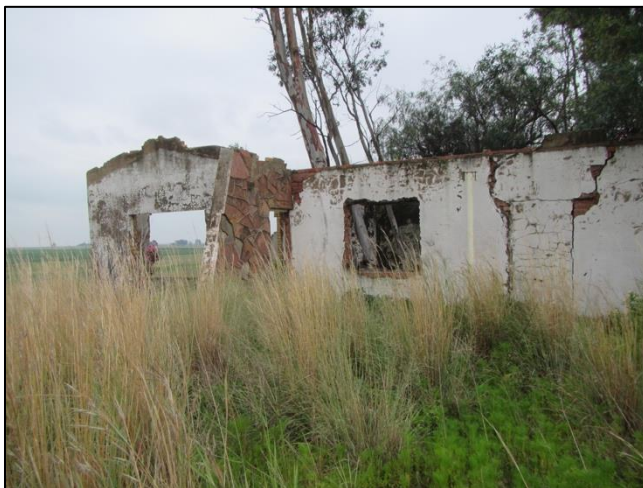
Figure 20 – MN004 dilapidated farm house
