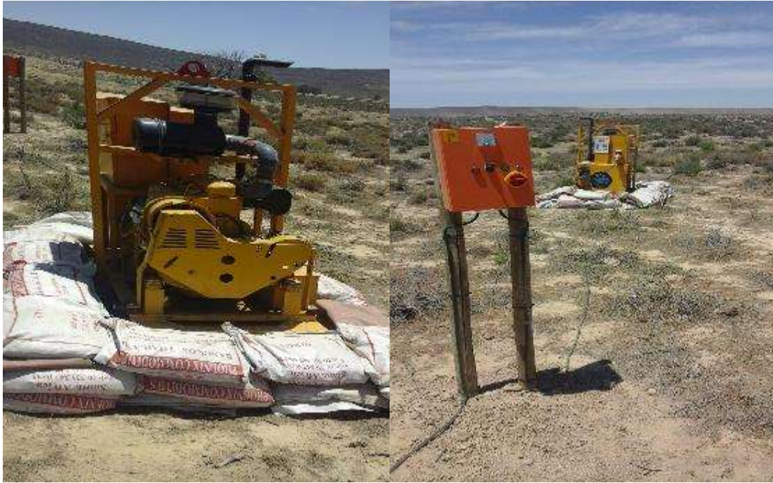
Figure 14: Installed water pump with electrical backup for abstracting water from the dam.
