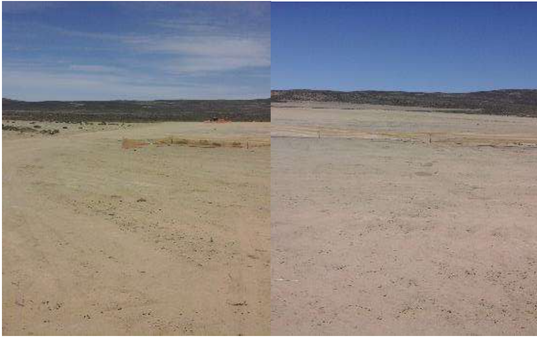
Figure 8: View of project site camp location within the project footprint being cleared.
