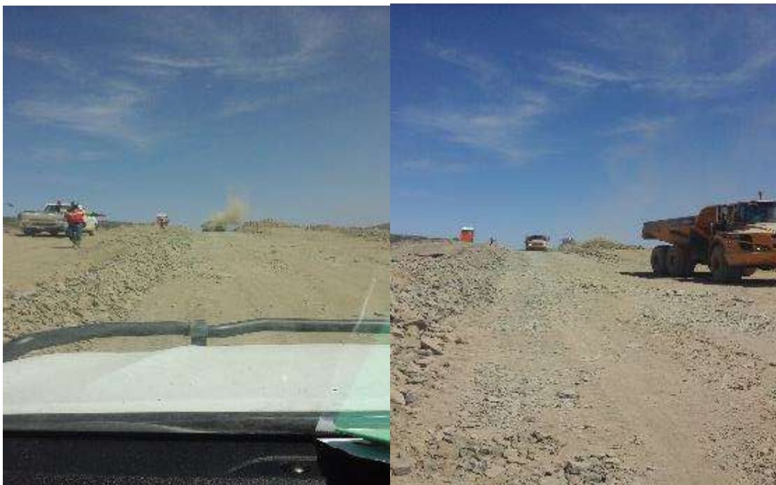
Figure 7: Traffic control being implemented where construction vehicles are at work to avoid accidents.
