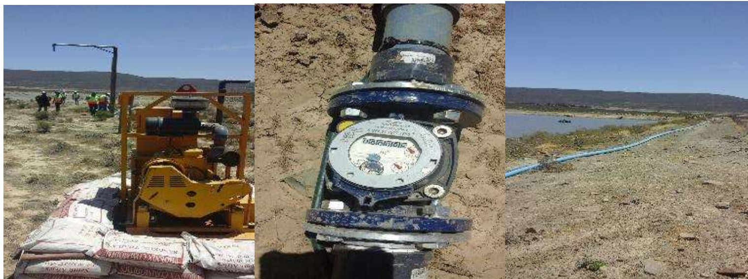
Figure 5: Installed water pump, flow meter and conveyance pipe for water abstraction from the dam.
